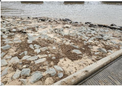
No north seep
