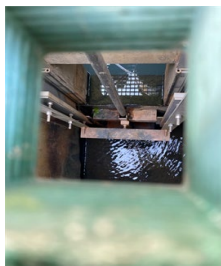
Inside effluent cell, just dip of water flowing
