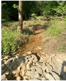
End of rock, standing water near rocks.
