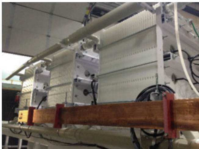
Flow Battery Energy Storage Unit
