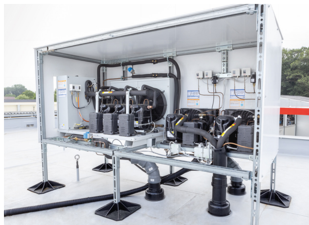
R-1234yf centralized system and two stand-alone LT units with R-454C.
