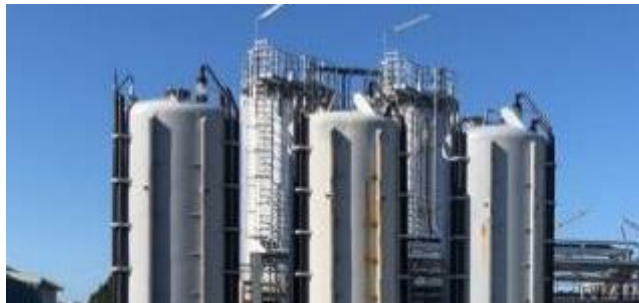
Final Step GenX Removal from Wastewater Dordrecht
