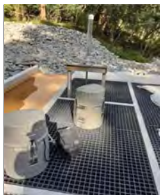
Seep D Effluent not bypassing
